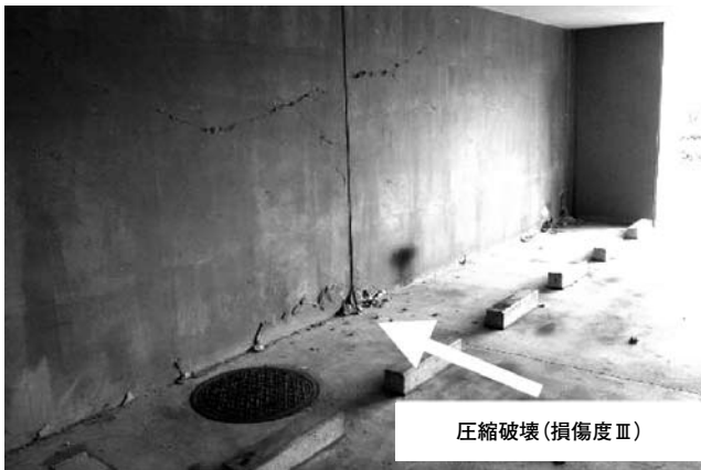
写真-6 耐震壁に生じた圧縮破壊
